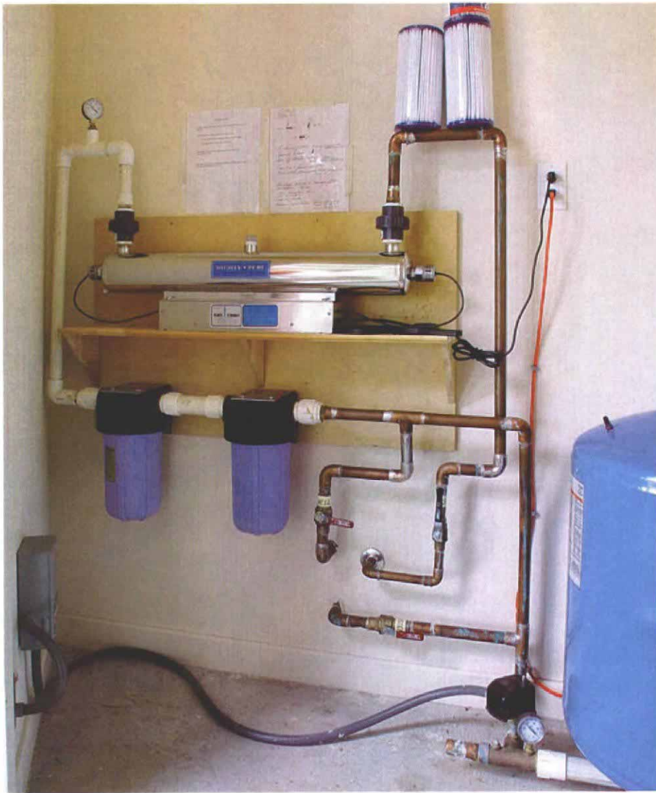
Next stop, your drinking glass. A submersible pump in the cistern sends water first to the pressure tank (far right in photo). The water then runs through a sediment filter (bottom center) and is purified in a UV-filter (top center).
